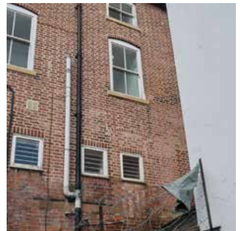
Evidence of previous openings
