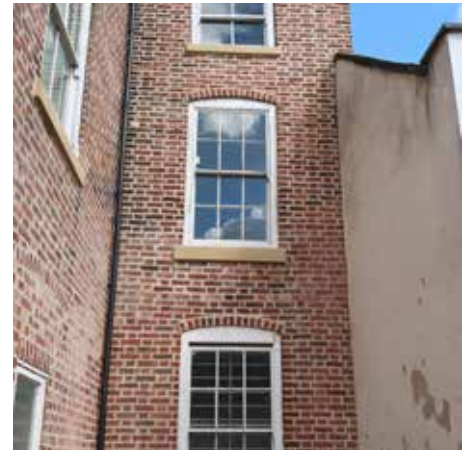
Evidence of replaced lintels
