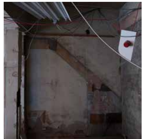
(ii) Evidence of lost stair (North)
